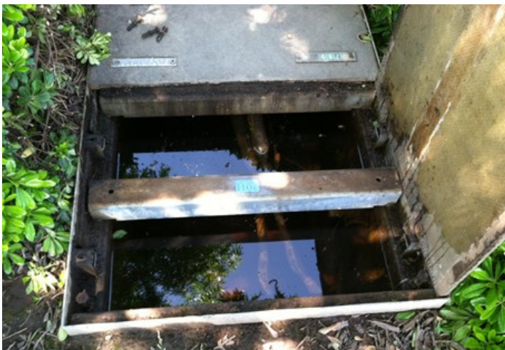
Underground utility enclosures filled with water and breeding mosquitoes.
